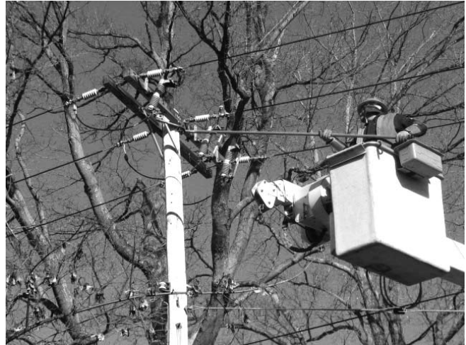
Truck Foreman Jay Willets installs a fuse
